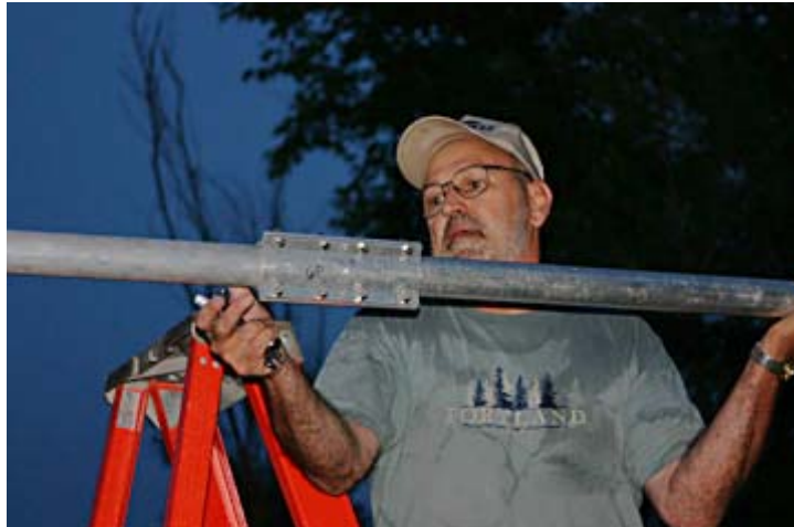
Charles, KC9DAO, checks the alignment of the big 40 meter rotating dipole during Friday night set-up.
